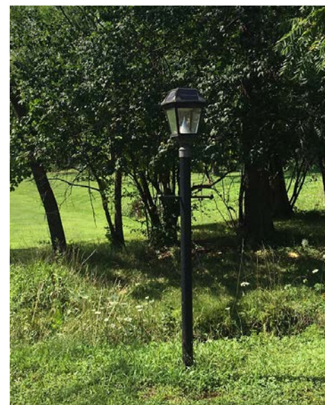
Existing pedestrian pole lighting
